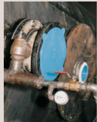
Testing All tanks are air tested for leaks at 5 psi. All seams are inspected to ensure weld integrity.
