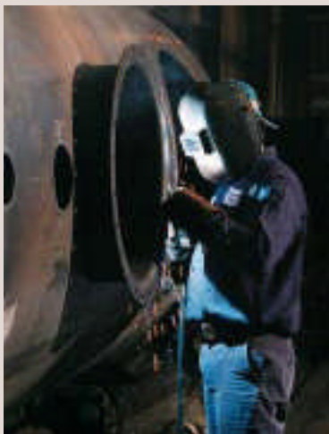
Fitting Components Manways, flanged and threaded fittings, coffer dams, and other special components are fitted to the tank, then welded in place.
